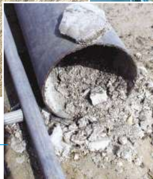
Deposits of CaSO 4 in a sludge pipe
